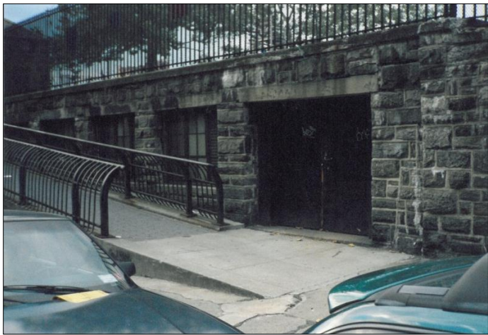
Figure 7. The door and windows of the storage room at John Jay Park.
